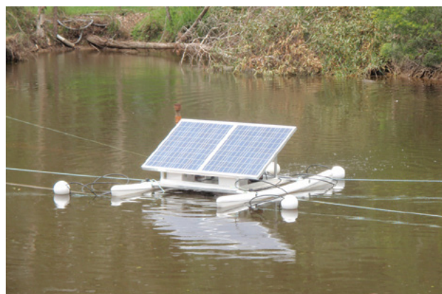
Figure 4.28 Solar water circulation system close up
