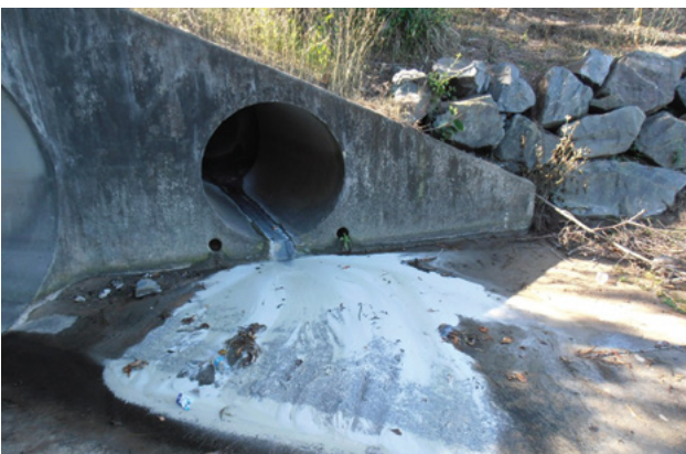
Photo: Colin Bridges, Gold Coast City Council
