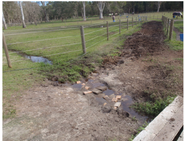
Figure 5.16 Before - gully crossing is eroded and degraded
