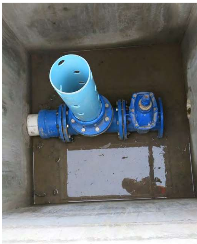
FIGURE 31 Photo outlet riser Photo: Shaun Leinster - DesignFlow
