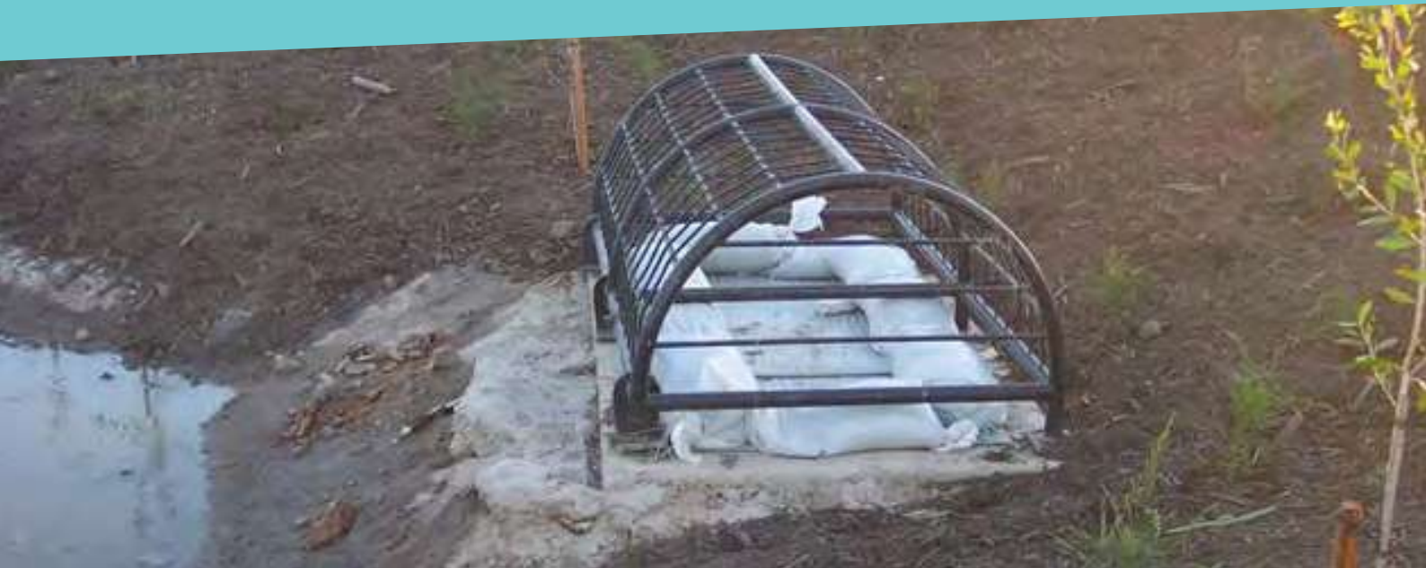
FIGURE 23 Photo Overflow pit blockage and flow diversion
