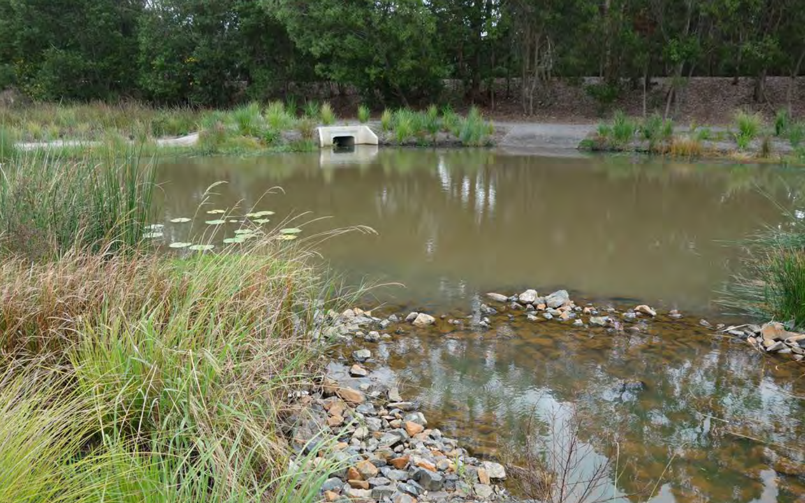
FIGURE 19 Sediment basin pipe connection only
