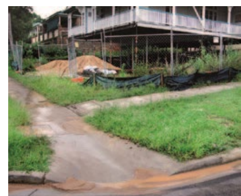
Sediment from building sites is a form of pollution that can deliver sediment and nutrients to waterways.
