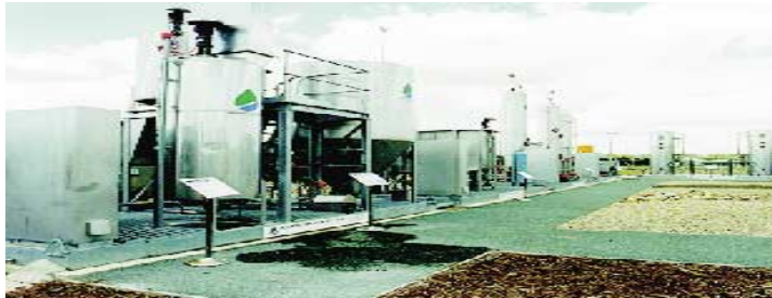
Advanced Water Recycling Demonstration Plant - Part of the Queensland Water Recycling Strategy Initiatives
