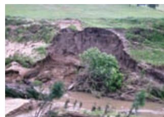
Erosion from January 2008 flood in the Logan and Albert catchments because of poor riparian management.
