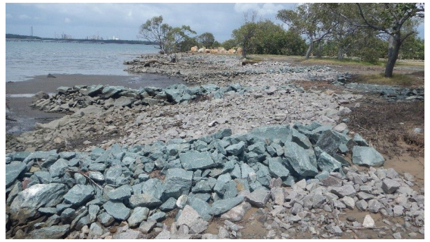
Rock groynes and rock beaching were constructed in the most susceptible areas.
