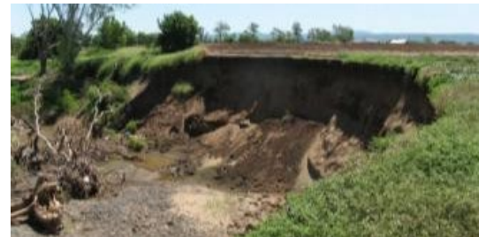
LOWER TENTHILL: Mass failure has resulted in a bank slump in the above example. This poses a serious safety risk to farm traffic and workers.
