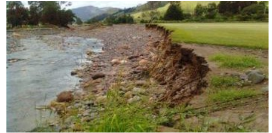
MT SYLVIA: Scouring has occurred here resulting in a very unstable steep bank, impacting on the productive potential of the farm.
