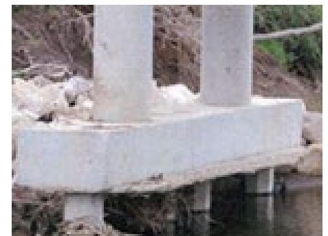
Streambed lowering impacts on structural integrity of man-made assets as well as the stability of streambanks.
