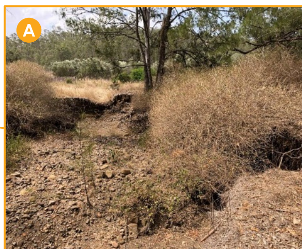
Figure 2. Aerial view of the erosion site before the erosion control work began. Inset A shows the erosion site looking upstream.
