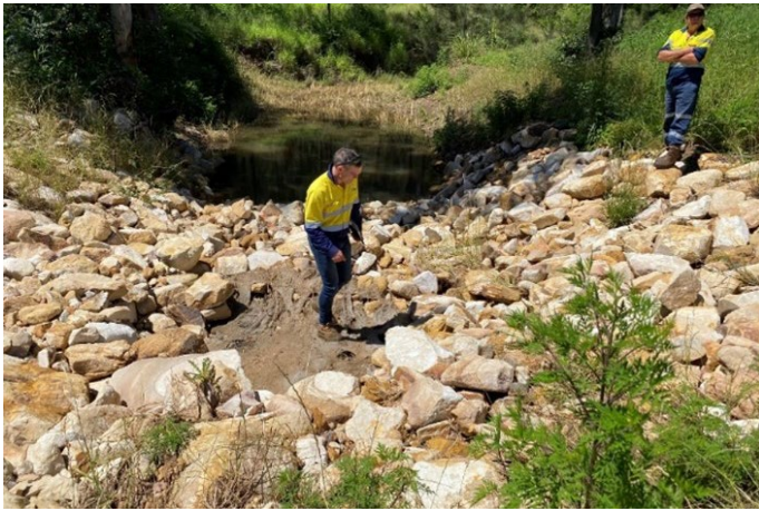
Figure 8. Some of the rock had been displaced during a rainfall event exposing the underlying damaged geofabric and soil.
