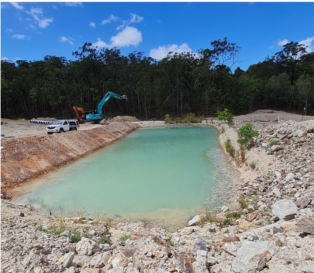
High efficiency sediment basin in a development site, Logan
