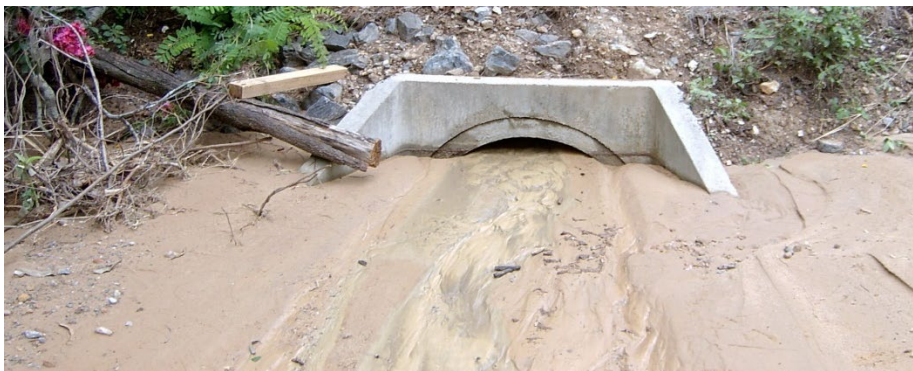
Sediment impacts on drainage infrastructure
